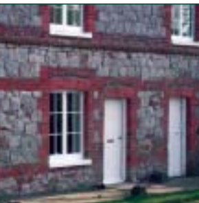
fig 43. Windows are small paned, with glazing bars painted white, typically with arched brick lintels over, although some straight lintels are also seen.
