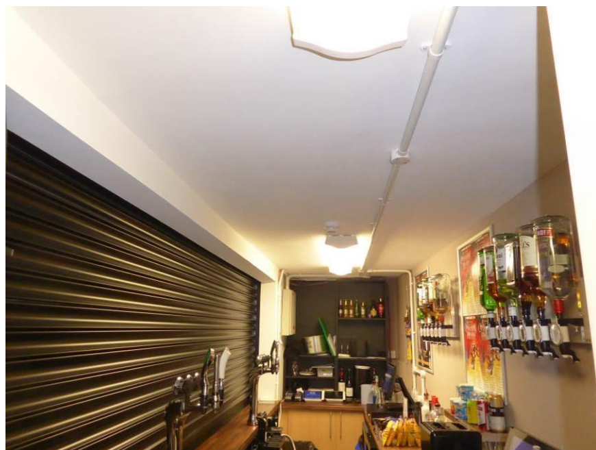
Photo 8 and 9 – ceilings over the Servery and the Kitchen.
