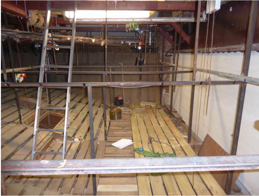
Photograph A17 – lighting platform over Auditorium, next to the stage.
