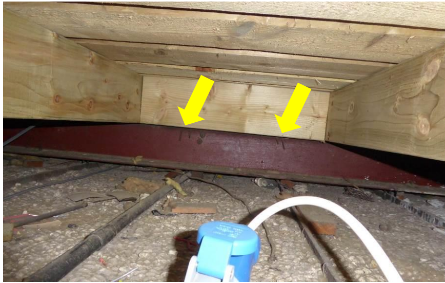
Photo 15 – metal wire ties hooked over the angle arm.
