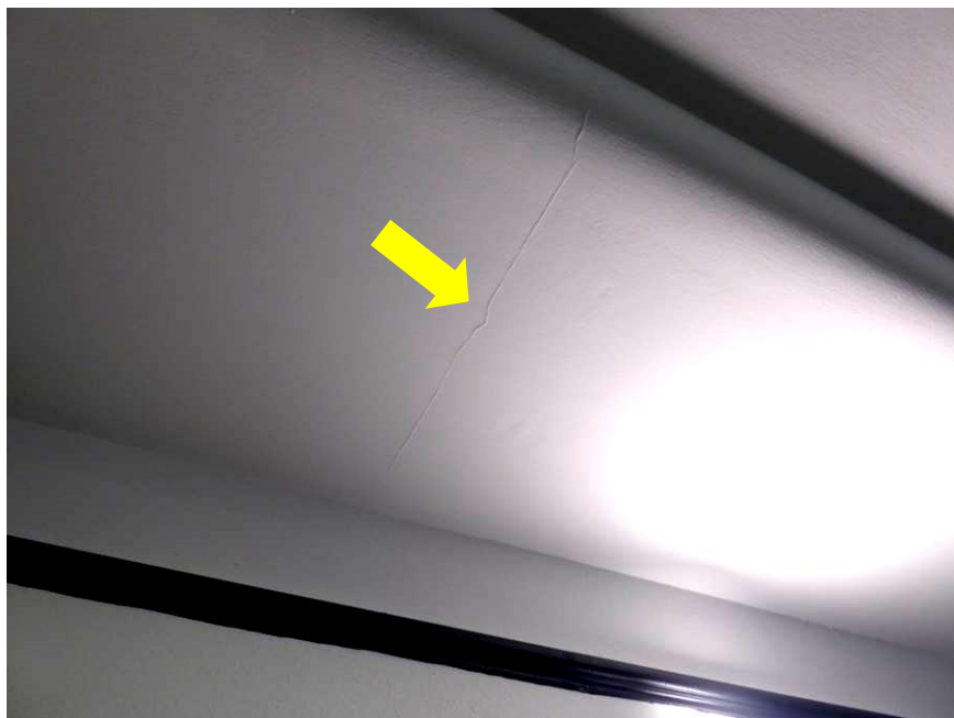
Photo 7 – crack in Foyer ceiling.
