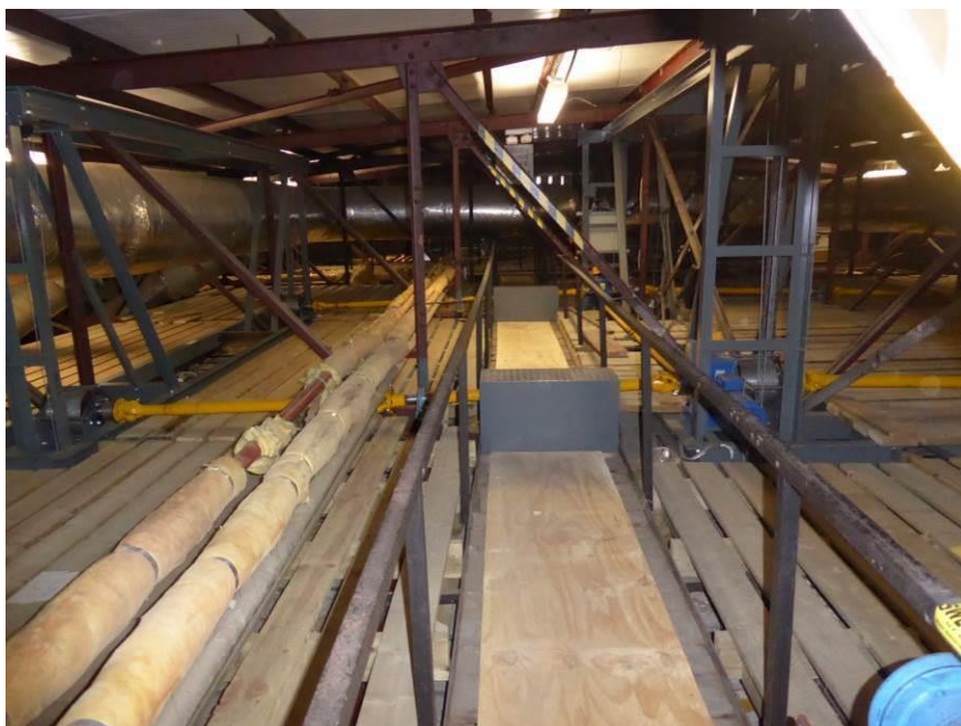
Photograph A16 – light box hoist over auditorium.
