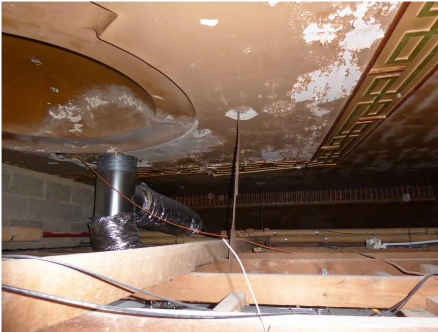
Photograph A19 – light box hoist over auditorium.
