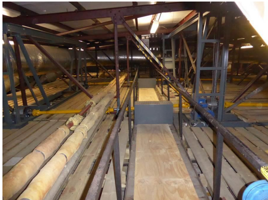
Photo 12 – services in loft above Auditorium.
