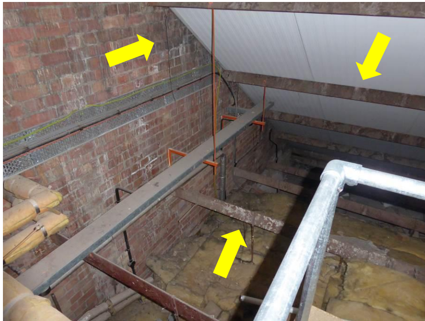
Photo 28 – staining on supporting angles (secondary beams and purlins) and wall.
