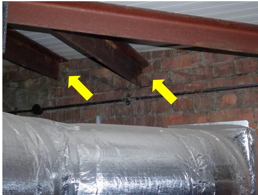
Photo 29 – surface corrosion of purlins bearing in external wall.
