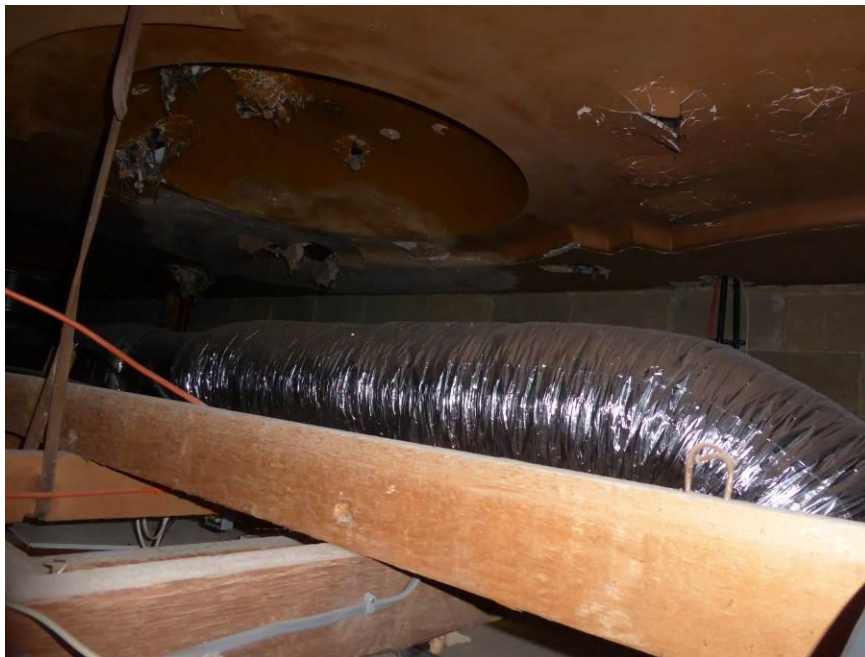
Photo 32 – damaged underside of the ceiling over the Alemein Room.
