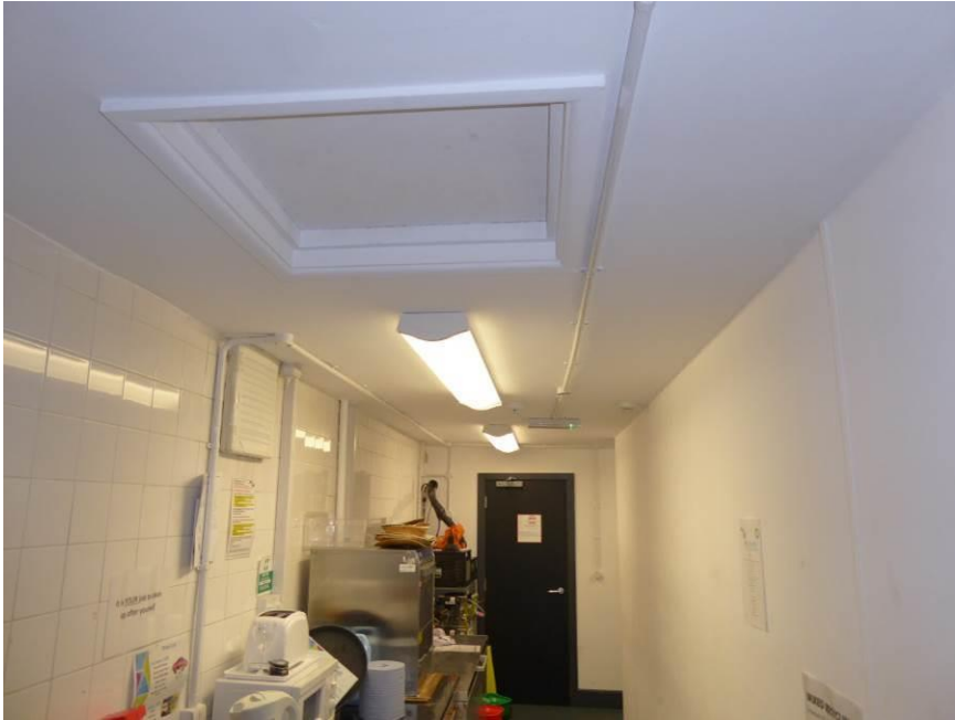
Photograph A9 – Kitchen ceiling.
