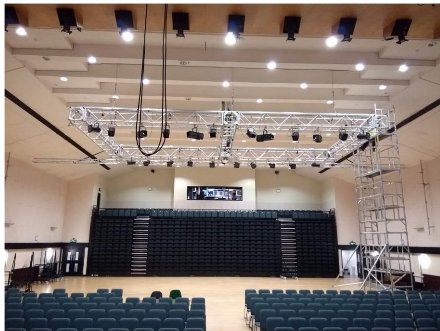
Photo 10 – Auditorium, retractable seating and light box.
