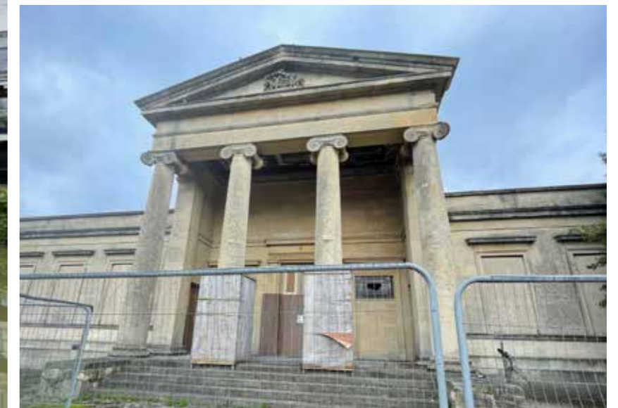
Assize Court will be restored and re-used as a key cultural destination containing a relocated Wiltshire Museum.
