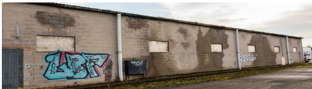
Below: Derelict buildings, Station Works
