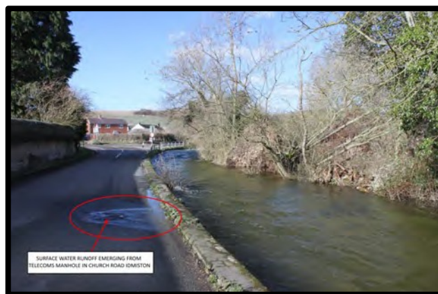
Surface runoff water forcing its way OUT of telecoms ducting at Idmiston
