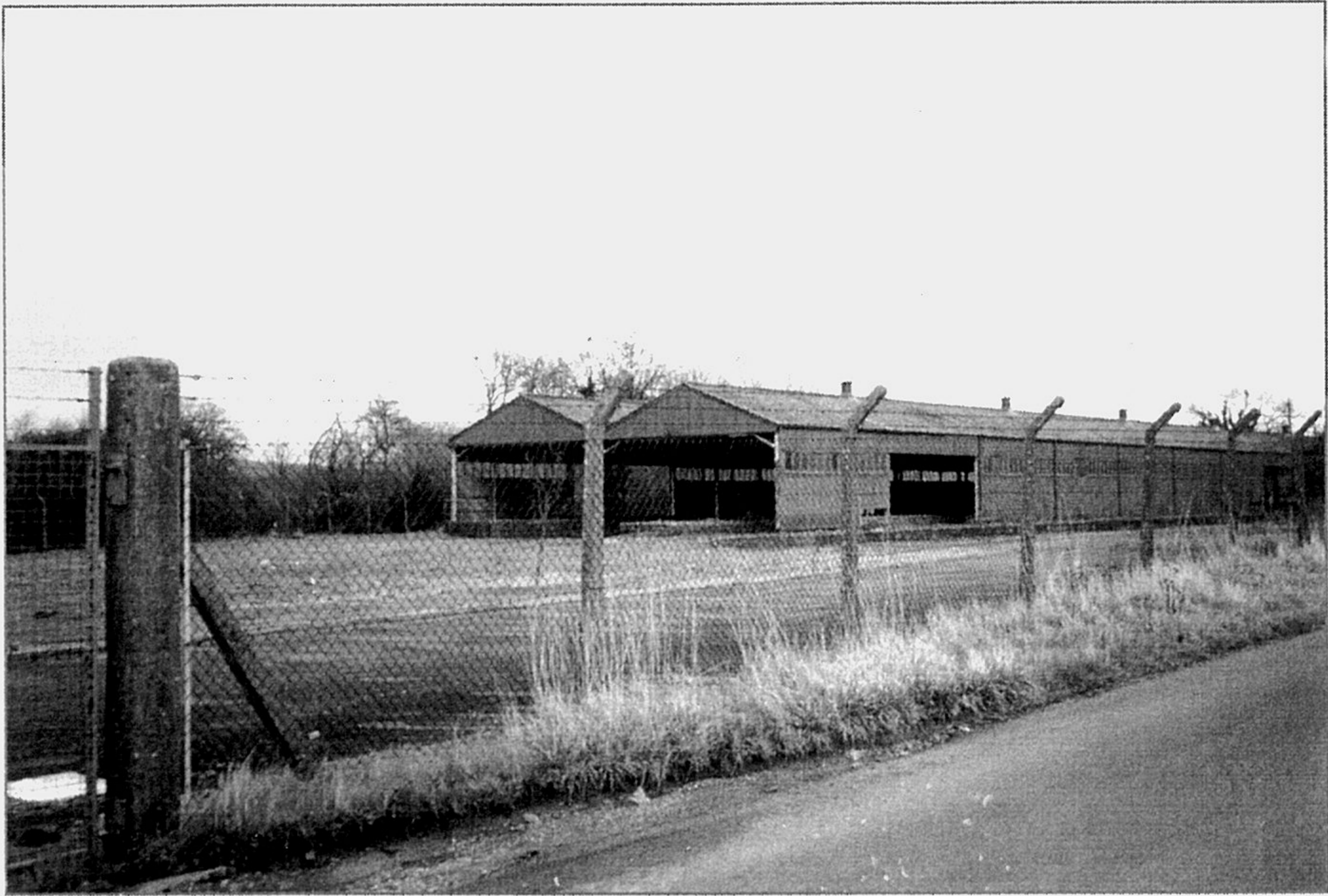
G. The transfer station in EM Valley is in poor condition structurally.
