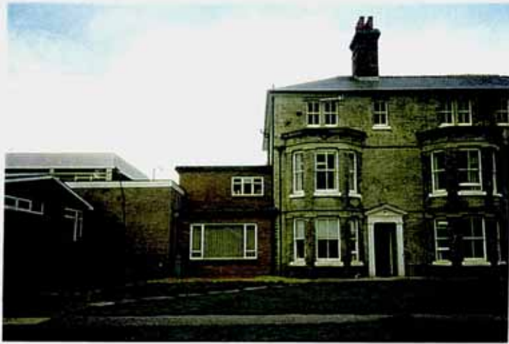
Southern elevation of Finch House showing inappropriate extensions.
