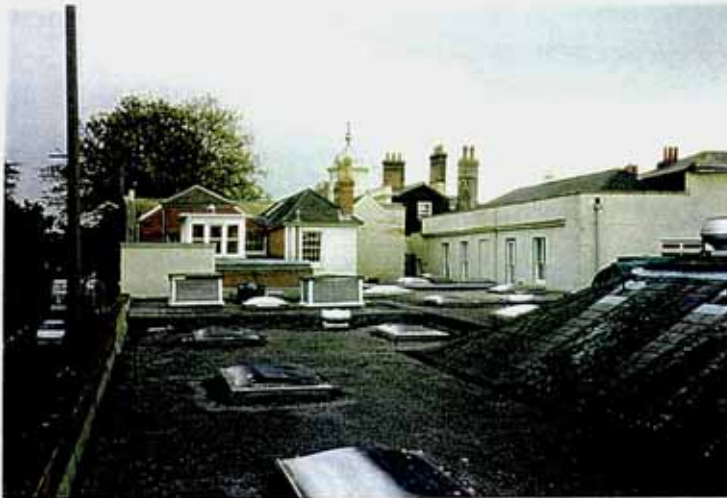
Many of the extensions to the Listed Buildings are inappropriate and should be removed.
