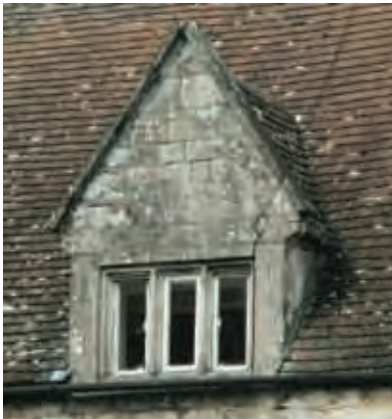
Medieval stone gable with parapet gable. Stone mullioned window, original leaded casements have been replaced.
