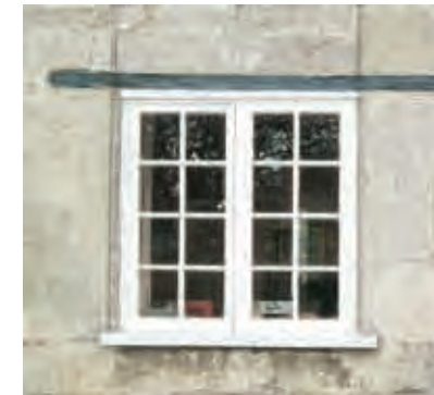
Casement window with timber lintel. Length of lintel suggests windows have been modified at some stage.
