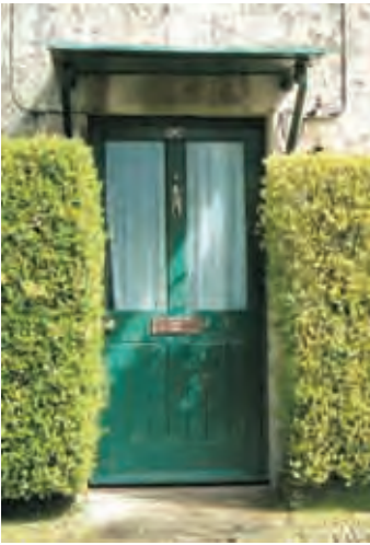
Very simple timber canopy on iron brackets, well suited to cottage form.
