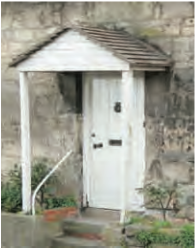
Projecting tiled, pitched roof canopy to cottage is suited to cottage form.
