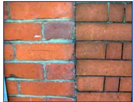
A crude junction between brickwork and mathematical tiles
