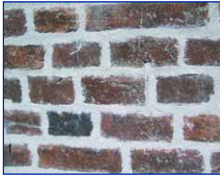
Poor brickwork with mortar joints that are messy, too wide and not tooled-in properly
