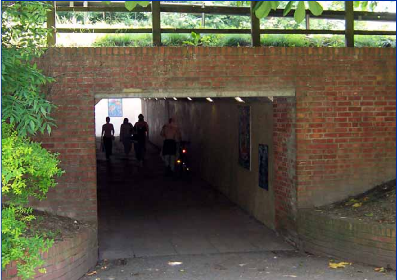
A poorly lit pedestrian underpass can feel very threatening
