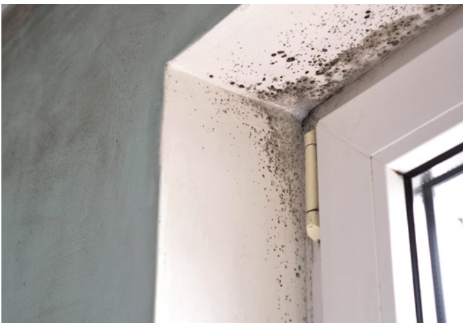
Signs of damp
