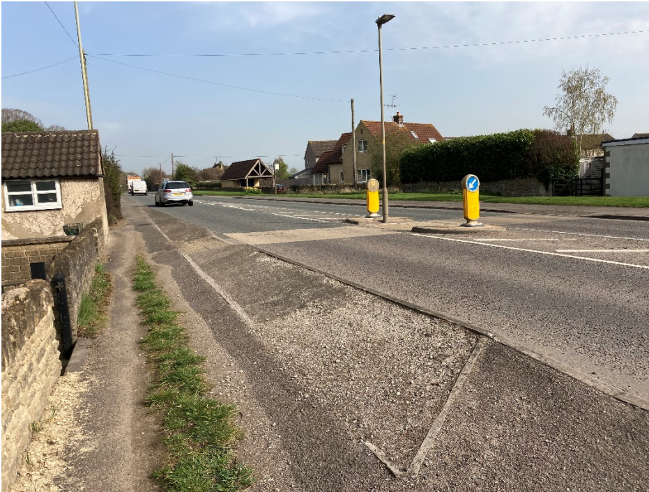
Figure 2-14 – A429 footway opposite Seagry Road with defects and considerable camber
